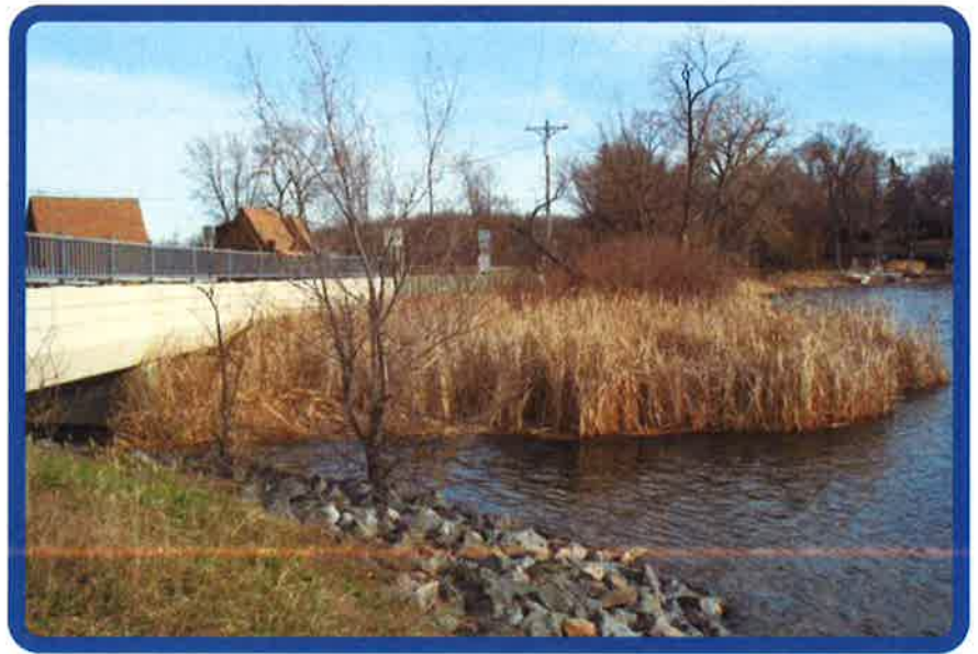
Floating bog blocking the Clearwater Lake outlet to Grass Lake at the bridge.
